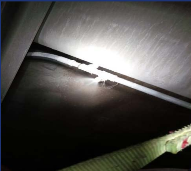
IN-SHAFT SYSTEM IN OPERATION
