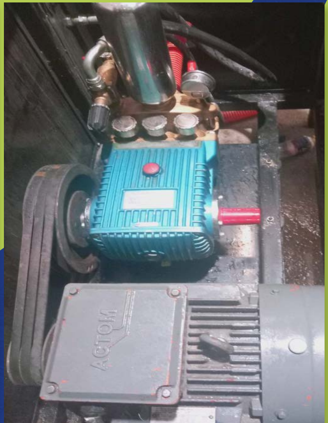
WL 160 PUMP STATION
