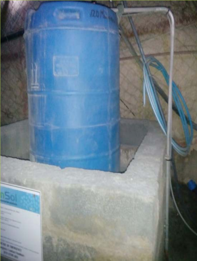
210 LITER CHEMICAL TANK IN BUND WALL
