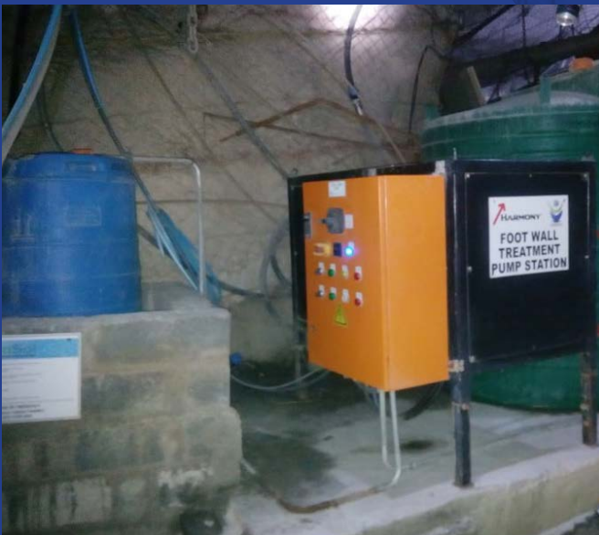
COMPLETE PUMP STATION AND DOSING PLANT
