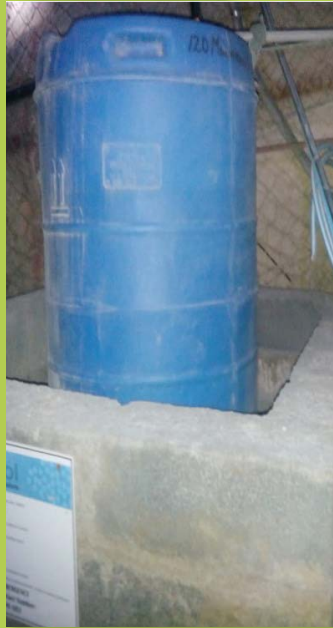
210 LITER CHEMICAL TANK IN BUND WALL
