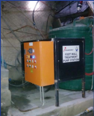
COMPLETE PUMP STATION AND DOSING PLANT
